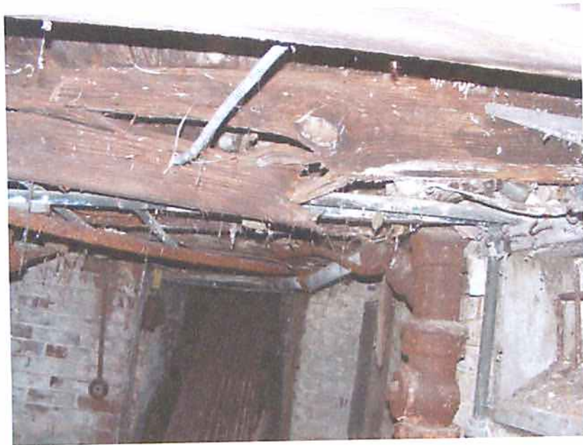
Photo M6 Structure #2234 - Collapsed First Floor Framing
