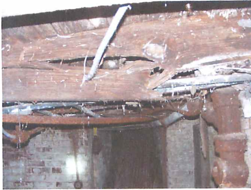
Photo M7 Structure #2234 - Collapsed First Floor Framing
