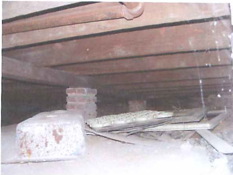
Photo L2 Structure #2228 - First Floor Framing Above Crawl Space- Shows Deflected Beams and Deteriorated Brick Piers and Brick Walls Beyond
