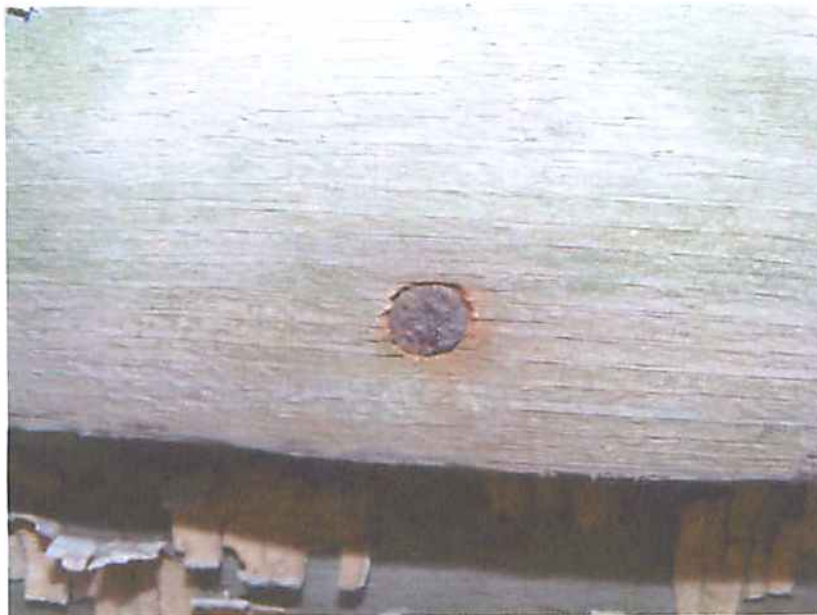
Photo M14 Structure #2234 - Rusted Nail Connection Wood Shingles to Exterior Stud Walls
