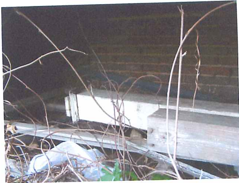
Photo M5 Structure #2234 - Deteriorate Exterior Face of Existing Brick Wall Below Porch
