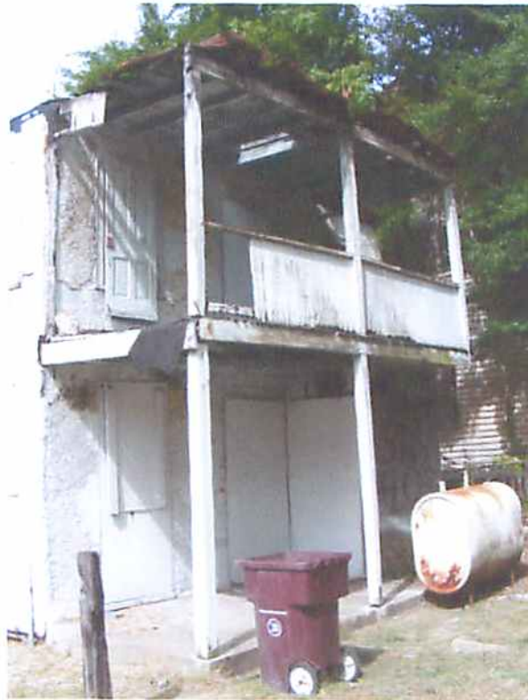
Photo R6 Structure #2238 - Rear Covered Porch - Corner Post Missing
