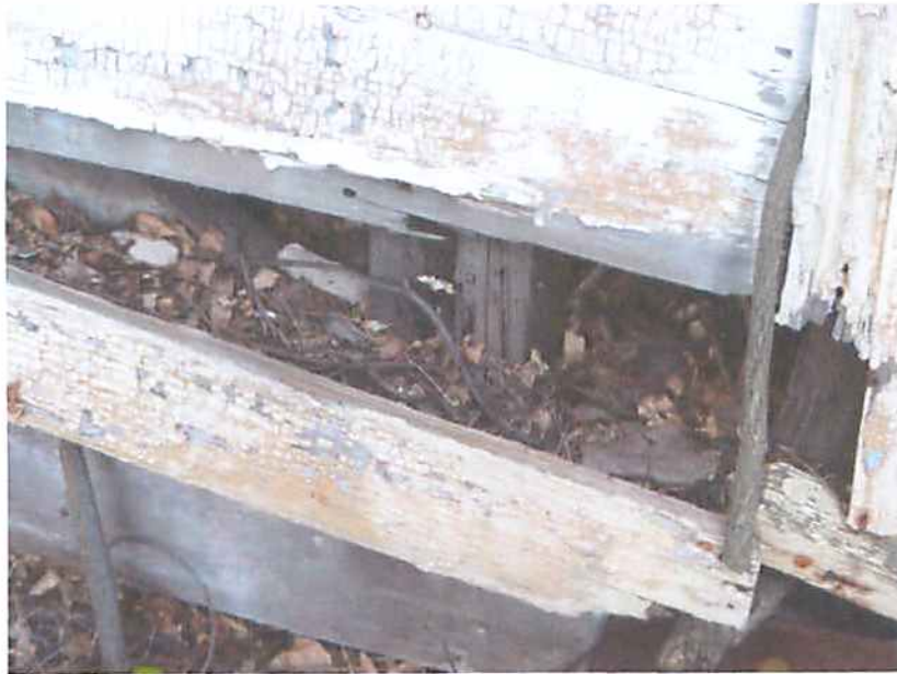
Photo L-16 Structure #2228 - Deteriorated Exterior Studs and Wood Shingles, Termite and Water Damage
