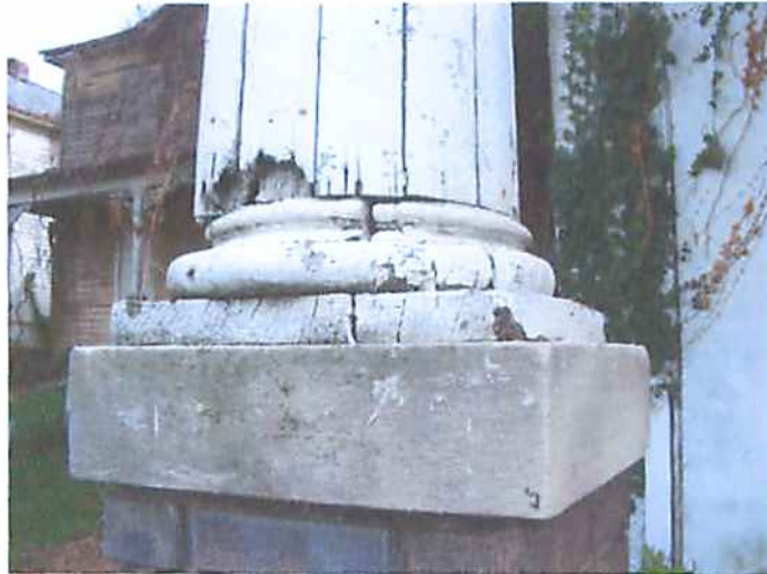
Photo R5 Structure #2238 - Base of Wood Porch Post Deteriorated- In Addition There is No Connection of the Column to the Pier
