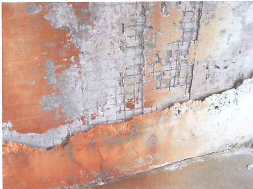
Photo R8 Structure #2238 - Typical Wall Covering - Wire Fabric Nailed to Wood Shingles Then Covered with Two Thin Layers of Cement.
