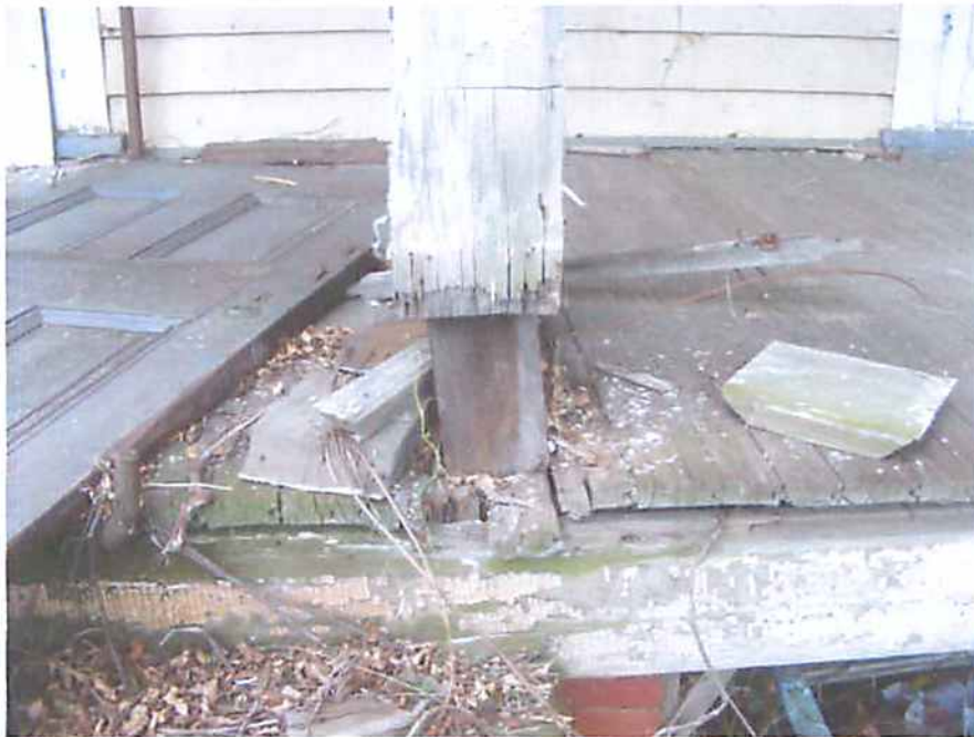
Photo M4 Structure #2234 - Failed Porch Post
