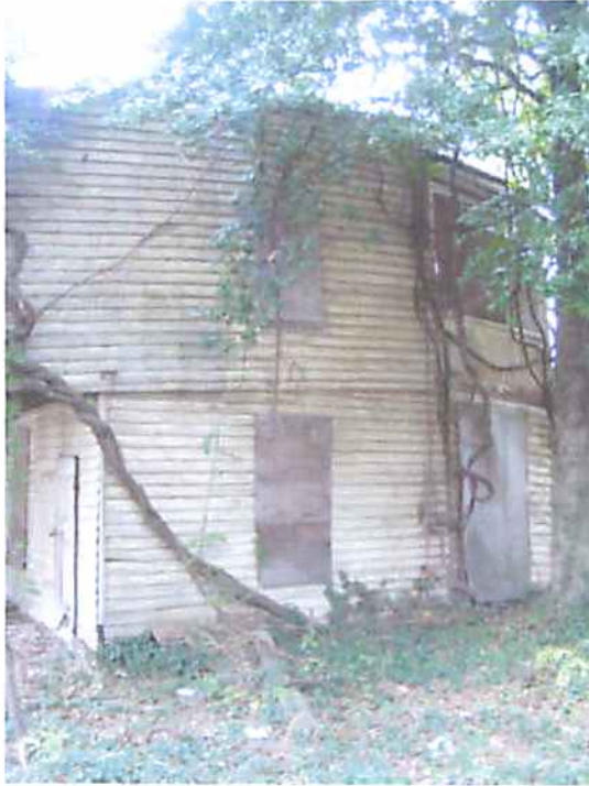
Photo M11 Structure #2234 - Exterior Wall of Collapsed Second Floor and Roof Framing at Rear of Building
