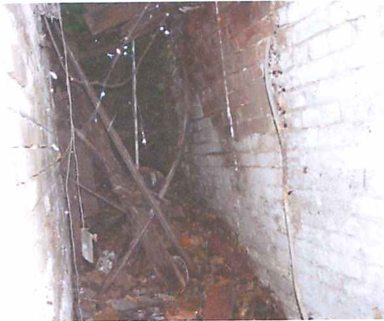
Photo L6 Structure #2228 - Shows Collapsed First Floor Framing at Access Stair in Basement
