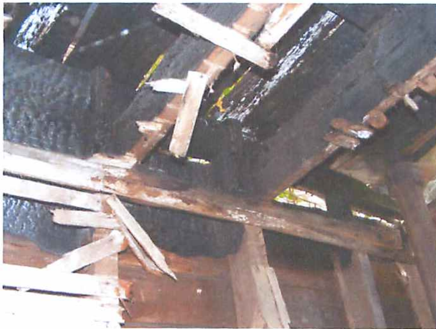
Photo R14 Structure #2238 - Fire Damage At Roof Level at Rear of Building
