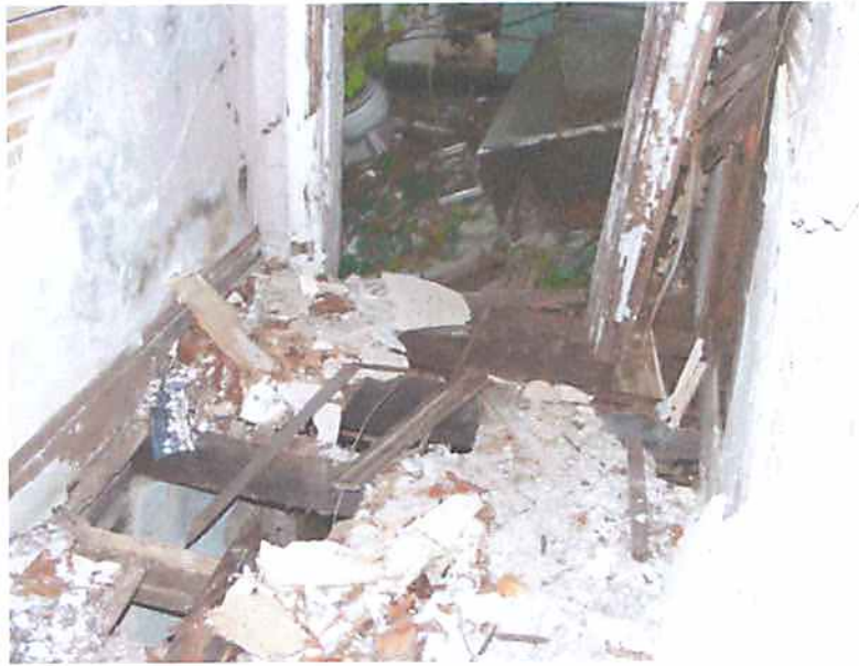
Photo L9 Structure #2228 - Shows Collapse of Second Floor Framing and Roof Framing Above
