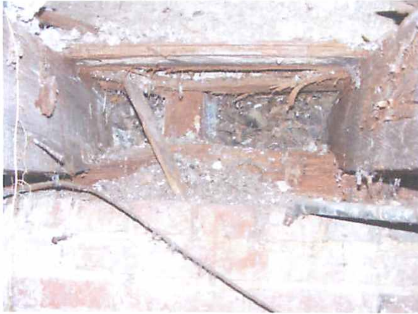
Photo M9 Structure #2234 - Damaged Wood Plate, Studs, Planking and Joists at Exteior Brick Bearing Wall
