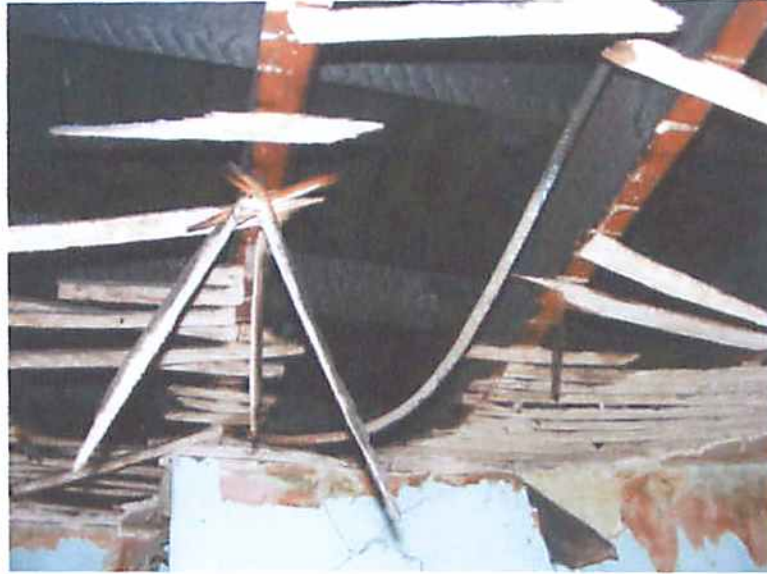
Photo R13 Structure #2238 - Fire Damage At Roof Level at Rear of Building
