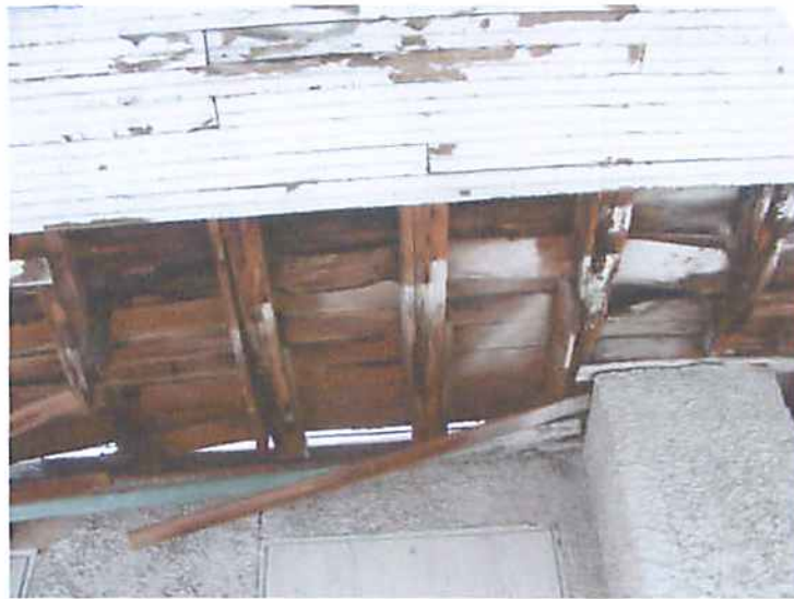
Photo R4 Structure #2238 - Shows Damage Porch Roof Framing
