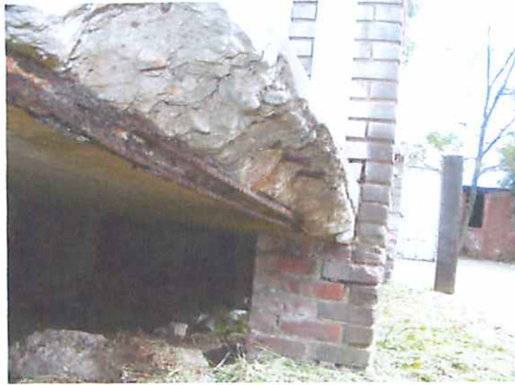
Photo R3 Structure #2238 - Shows Spalled Exterior Edge of Concrete Porch with Corroded Reinforcing Steel
