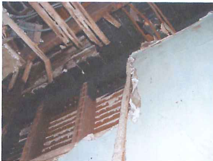
Photo M12 Structure #2234 - Interior Fire Damage to Ceiling and Roof Framing at Rear of Building
