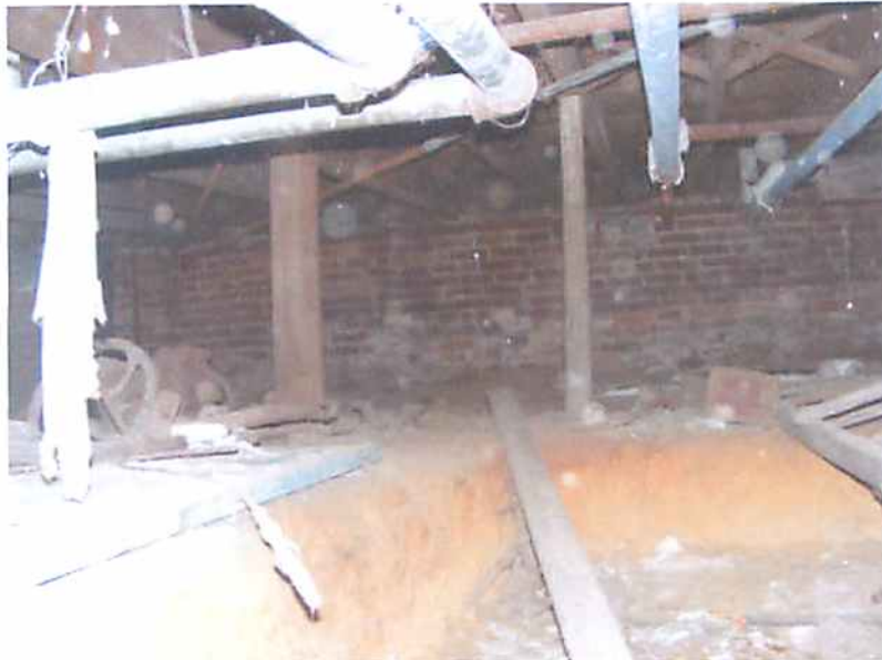
Photo M8 Structure #2234 - First Floor Framing Over Crawl Space - Post Used to Help Support Existing First Floor Joists
