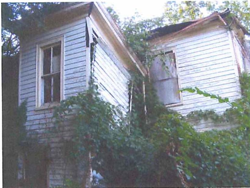
Photo L14 Structure #2228 - Collapsed Portions of Roof and Second Floor Framing at Rear of Building
