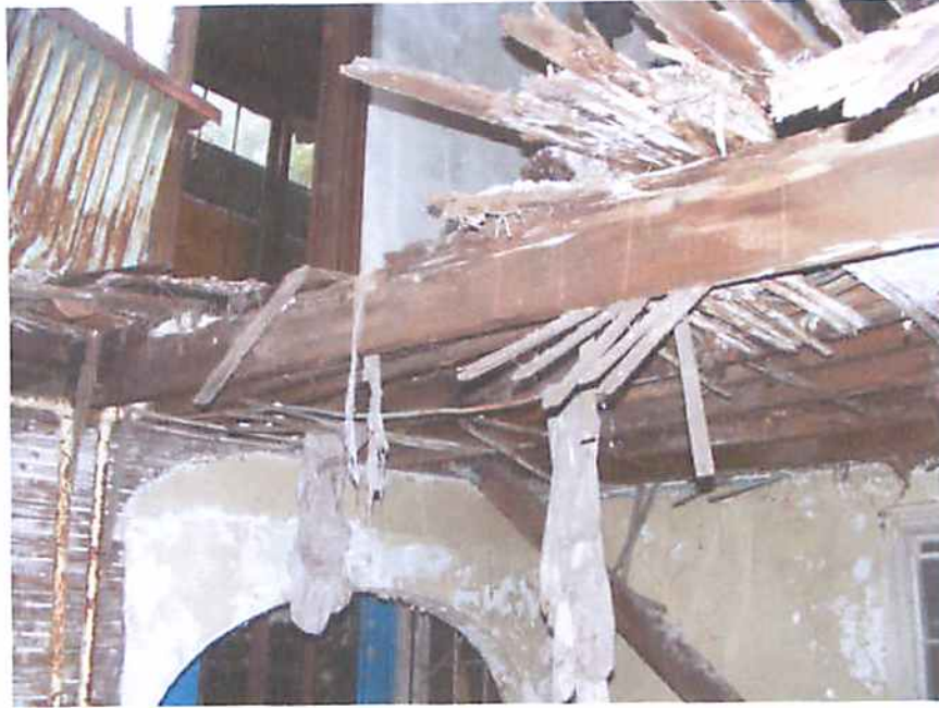
Photo M13 Structure #2234 - Collapsed Second Floor Framing
