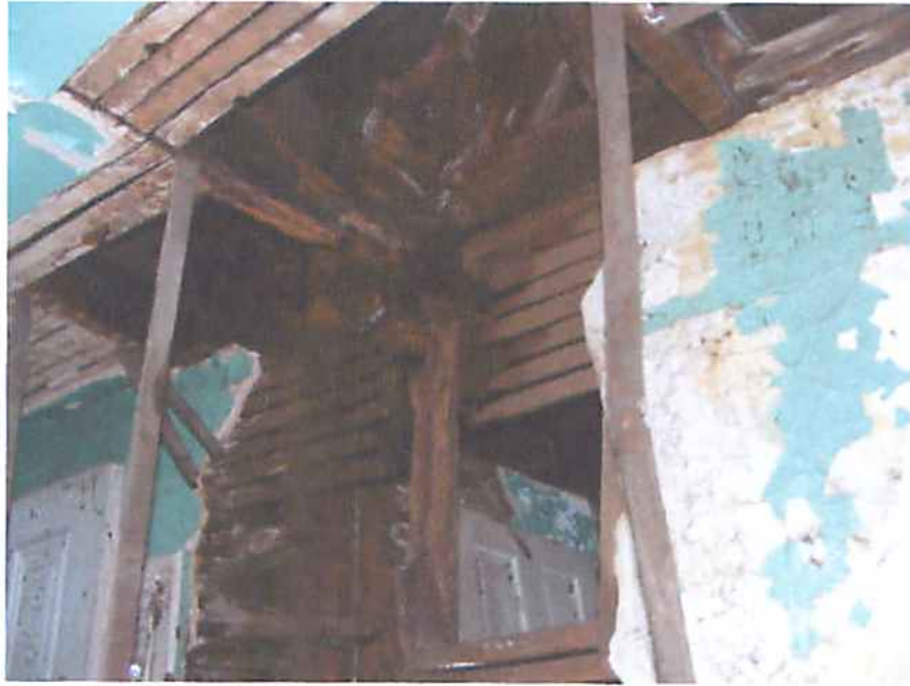
Photo L11 Structure #2228 - Shows Collapse and Deteriorated Roof Framing
