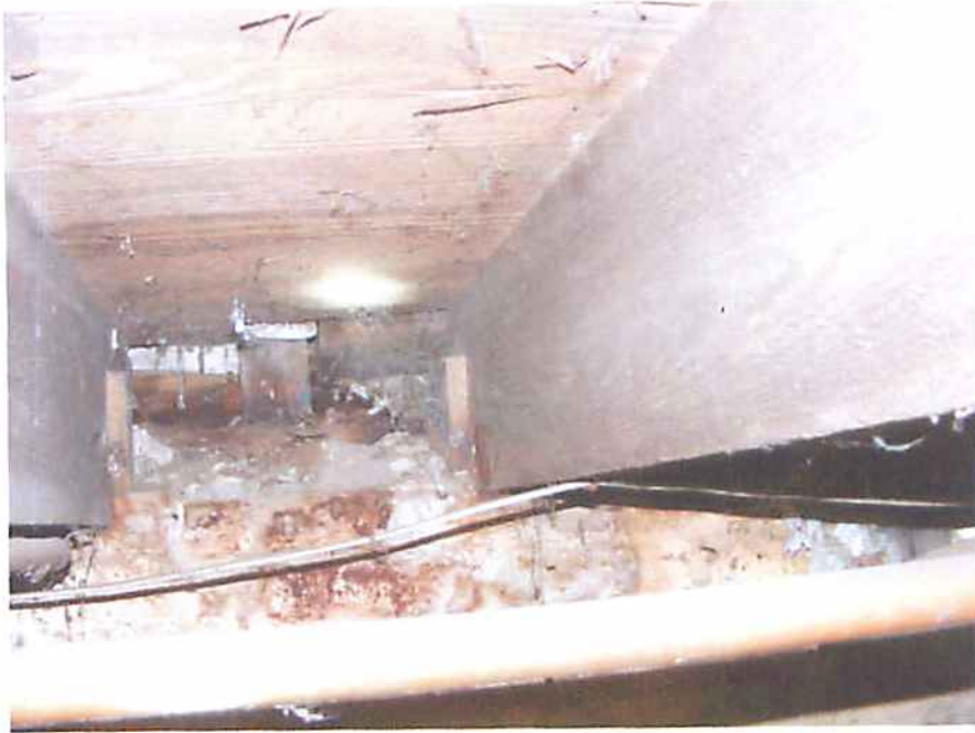
Photo R11 Structure #2238 - End Bearing of Existing First Floor Joists. Shows Deteriorated Wall Studs, Wood Plate and Joists
