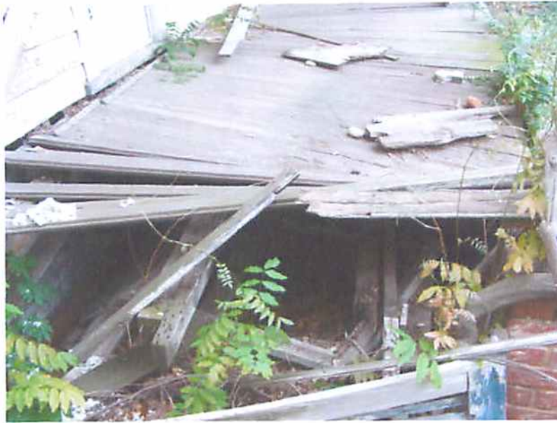
Photo M3 Structure #2234 - Collapsed Porch
