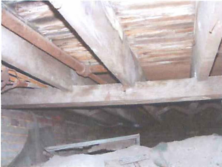
Photo L3 Structure #2228 - Shows Water Damage to First Floor Planking Above Crawl Space
