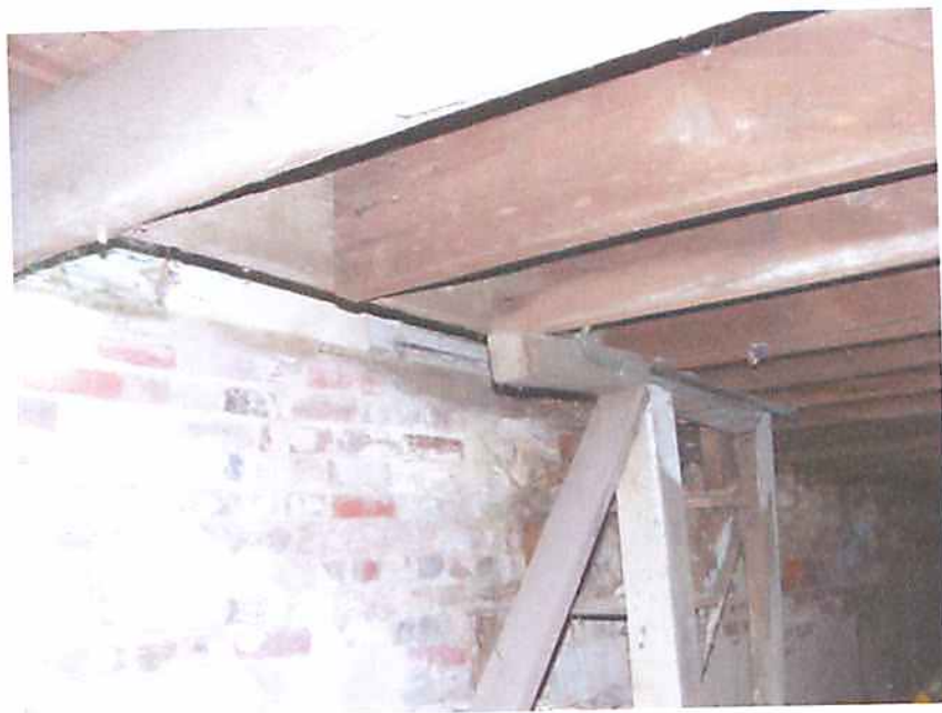
Photo R9 Structure #2238 - First Floor Framing Around Stair Opening - Deflected and Failing.
