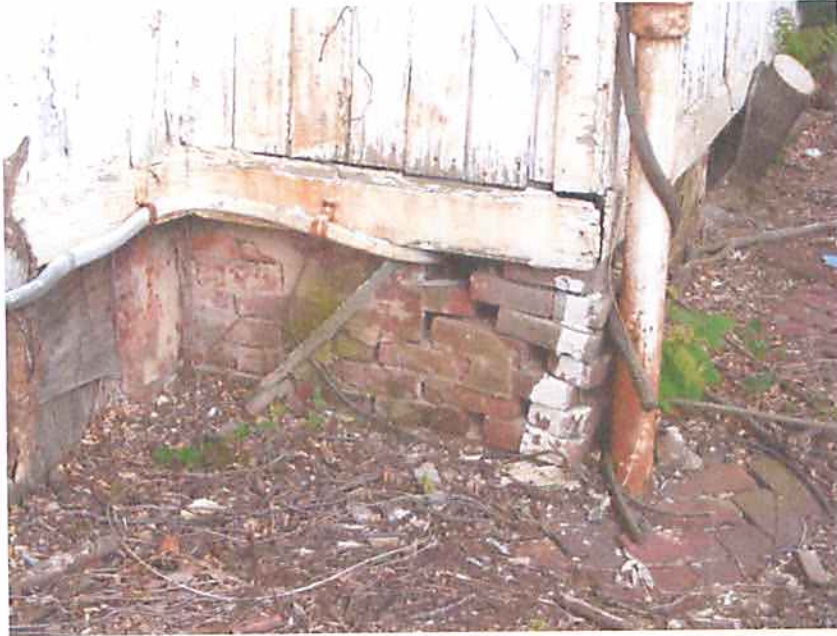
Photo L13 Structure #2228 - Collapsed Exterior Brick Wall
