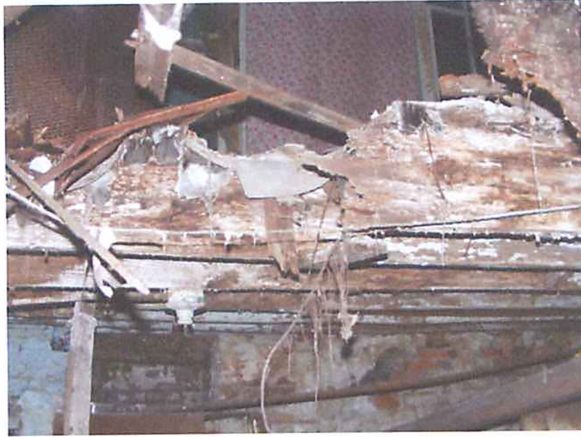
Photo L5 Structure #2228 - Shows Collapsed First Floor Framing
