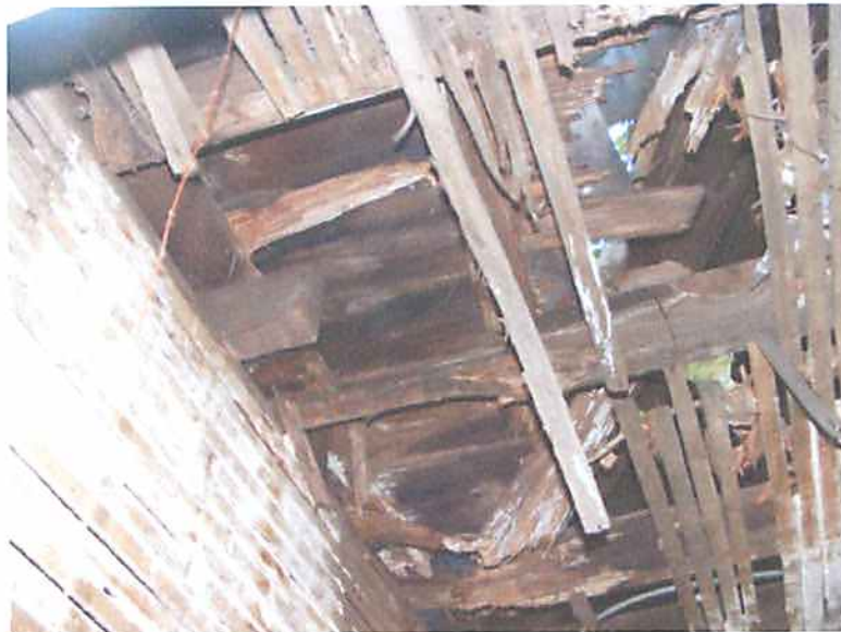
Photo L10 Structure #2228 - Shows Collapse of Roof Framing Above
