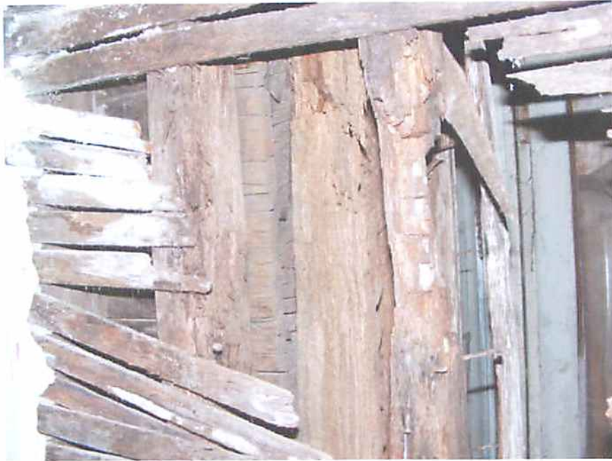
Photo L15 Structure #2228 - Deterioration of Interior Bearing Stud Wall Between First and Second Floor
