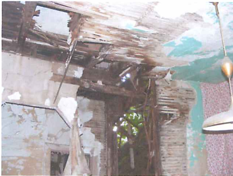
Photo L8 Structure #2228 - Shows Collapsed Second Floor Framing and Collapsed Exterior Bearing Walls
