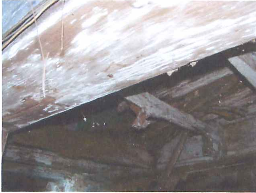
Photo L7 Structure #2228 - Shows Collapsed First Floor Framing Above Crawl Space
