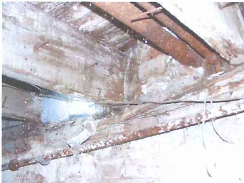
Photo L4 Structure #2228 - Shows Typical Deteriorate Wood Plates, Joists, Planking and Studs at Exterior Walls in Basement Area
