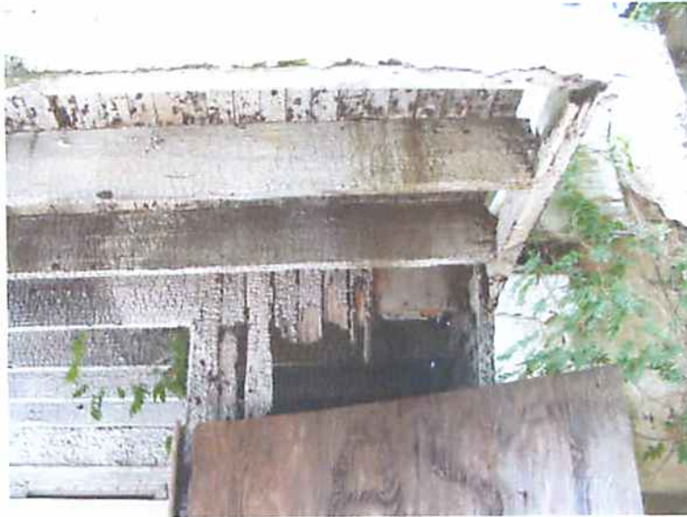
Photo R7 Structure #2238 - Second Floor Framing of Exterior Deck. Deteriorated with Fire Damage.
