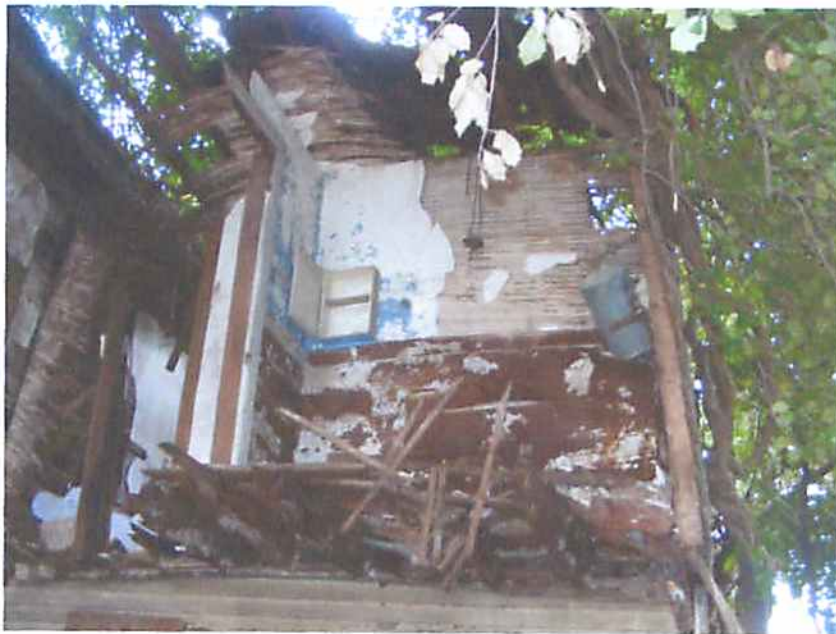
Photo M10 Structure #2234 - Collapsed Second Floor and Roof Framing at Rear of Building
